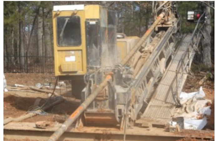
A drill rig is used for boring or directional drilling installation. It hollows out a space below ground that the pipe is then pulled through. Sections or "strings" of pipe are lined up in the easement or right-of-way as part of the installation process. The size of the rig varies depending on the size of the pipe and the length of the section being installed.
